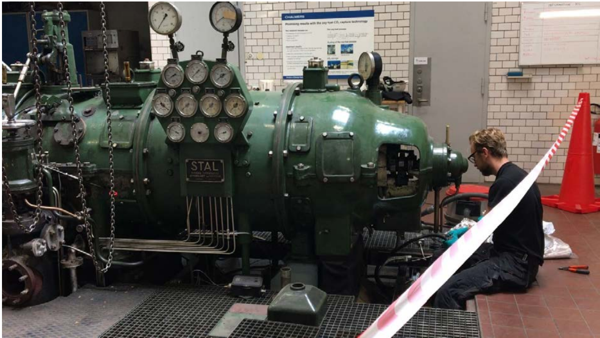
Icon of the project, the refurbished steam to electricity unit
